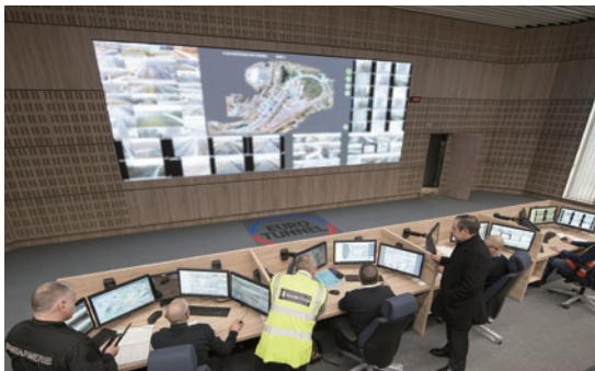
Eurotunnel New Security Control Center, French
